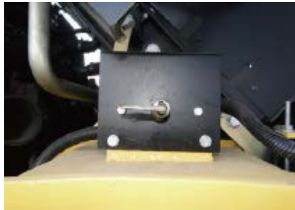
Fig. Engine compartment 1. Battery disconnect
