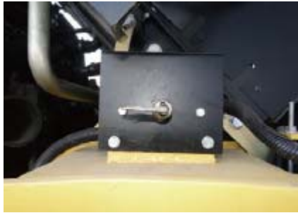
Fig. Engine compartment 1. Battery disconnect
