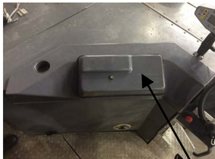
Fig. Example of panel protection
