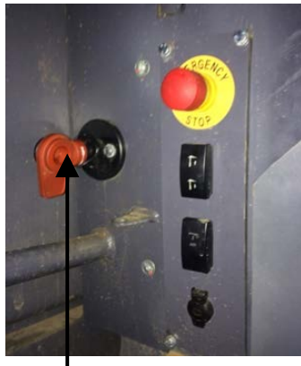
Fig. Battery disconnecter
